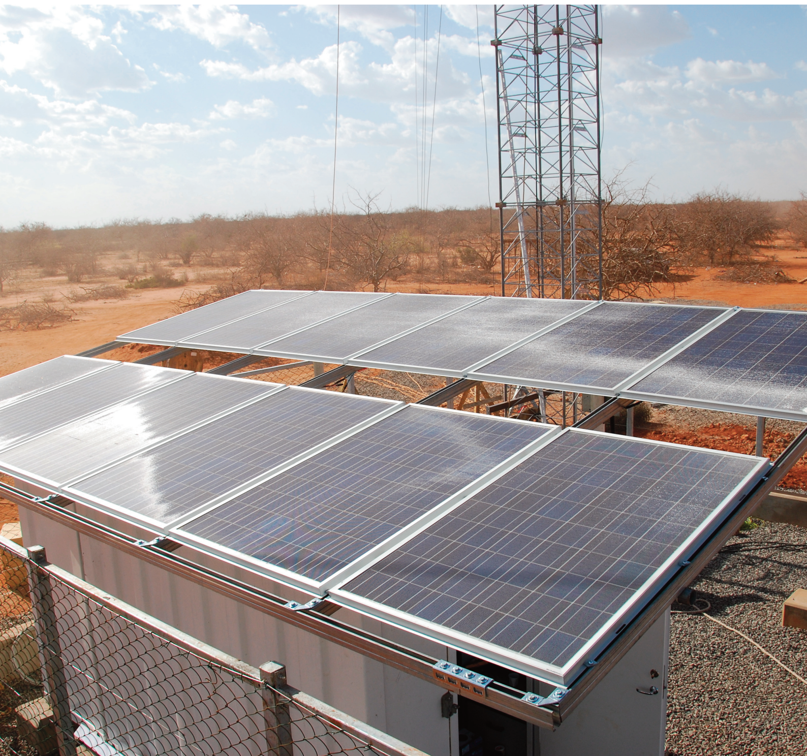
Image 7: Solar Energy Installation in Mozambique
